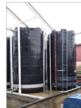
SMM's rainwater tanks
