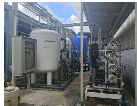
SATL's water recycling equipment
