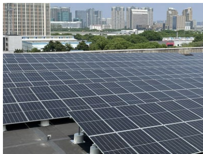
Solar power system installed on the factory roof
